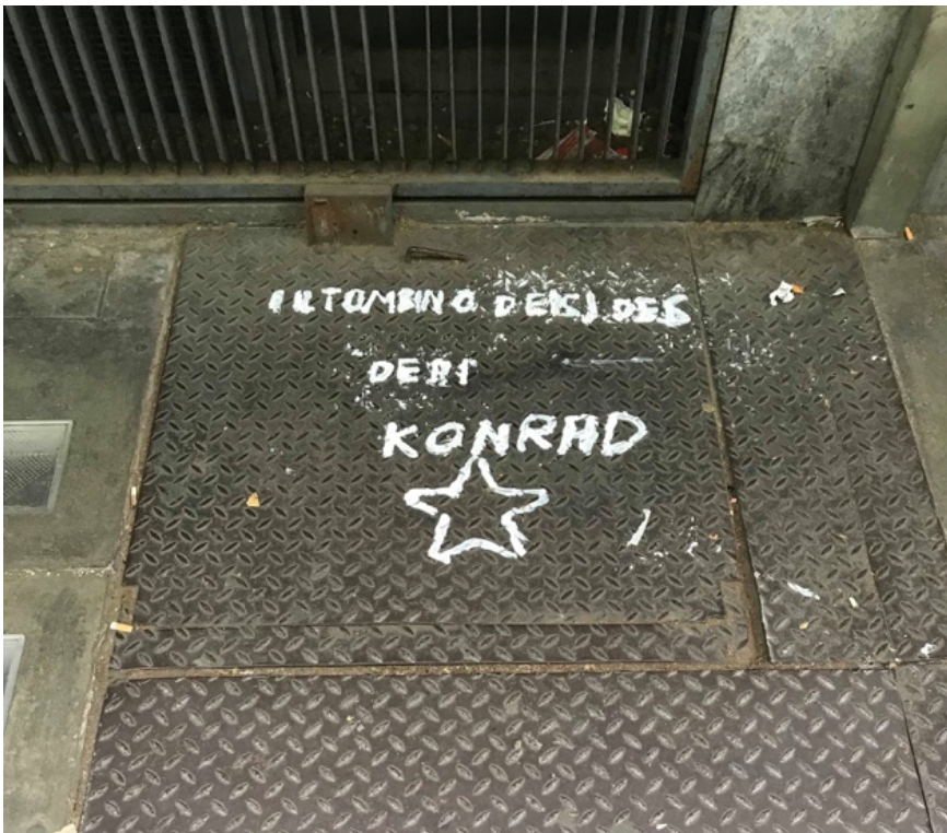
PHOTO 7: The manhole cover where the building's electrical system is found. After that night, it has been 'patrimonialized' by squatters as a place of worship (Photo by Chiara Cacciotti)
