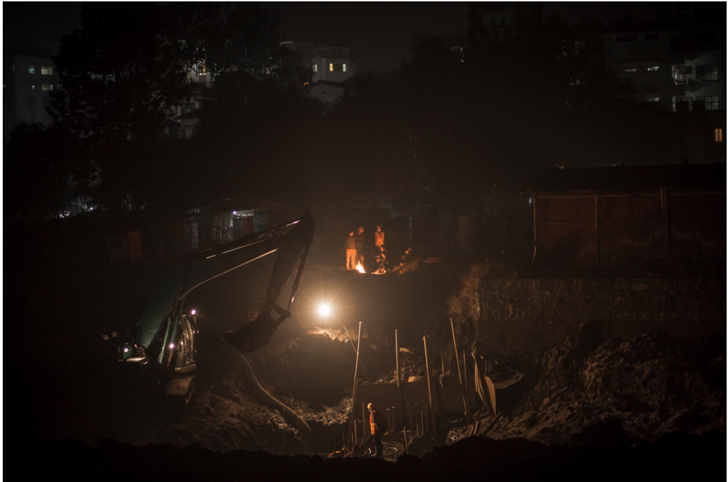
PHOTO 9: There are no fixed working hours in Kathmandu's construction sites. Sometimes labourers have to stay up to work in the middle of the night because of city regulations about the use of heavy machines.
