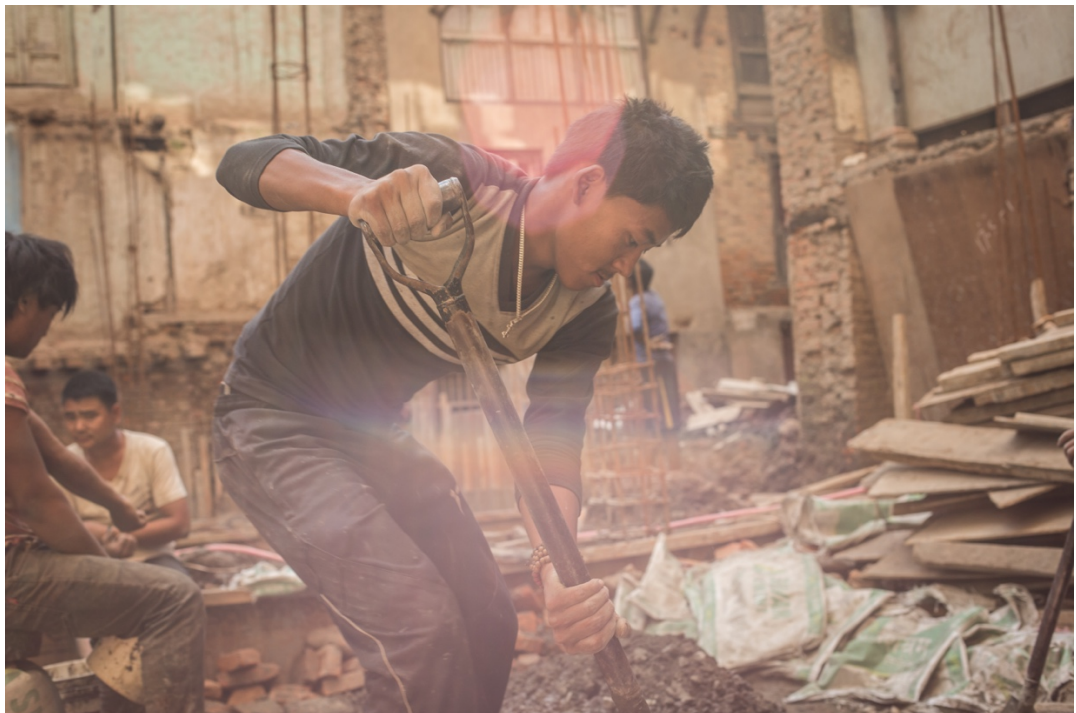
PHOTO 6: Carrying heavy loads and shovelling dirty are ‘entry-level’ jobs, for which no technical skills are required. The young men compete with one another to carry the heaviest possible load. Here, Dil, aged 19, shovels dirt in preparation for the construction of a new home that will replace a hundred-year-old residential building in Patan that was badly damaged by the 2015 earthquake.
