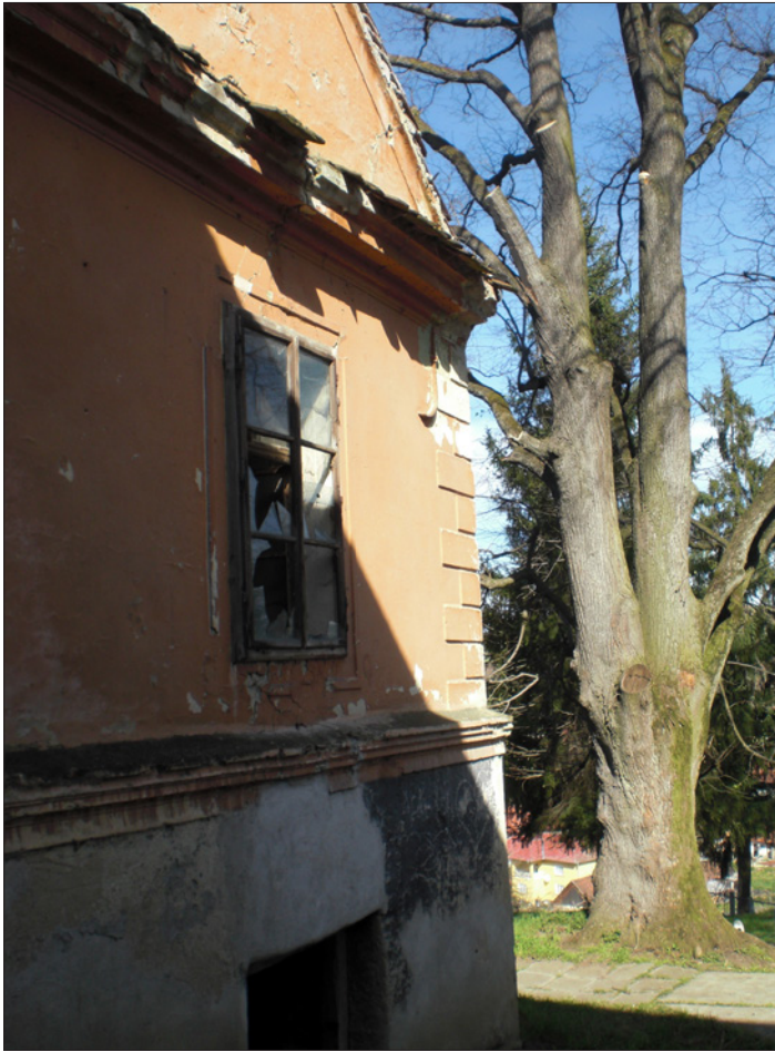
FIGURE 4 - BUILDING IN RUINS: THE BUILDING IN BURGBERG IS ABANDONED AND HAS BEEN ABOUT BY THE VILLAGERS, AND ALONGSIDE IT A PART OF THE HISTORY OF THE SAXONS. THIS IS SHOWN BY THE BROKEN WINDOW AND THE SHADOW THAT COVERS THE BUILDING. CRISTINA MONICA ANDREI, ASTRID PASCU.
