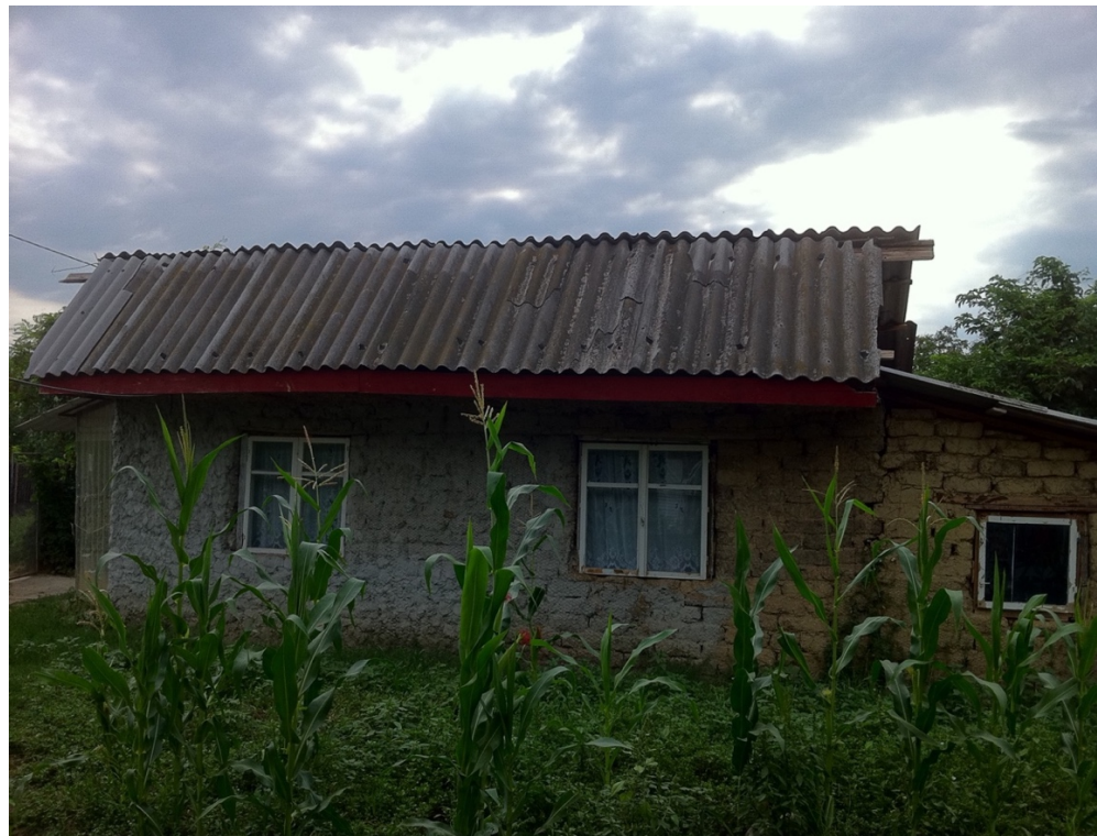
FIGURE 22: House in adobe with the roof redone in metal sheets before the migration
