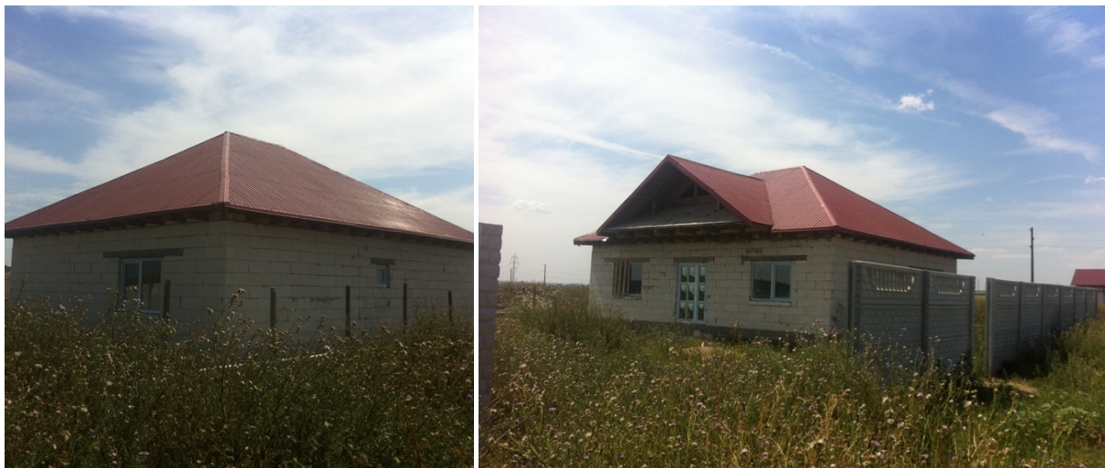
FIGURES 34-35: House under construction with the first and most important building phase underway
