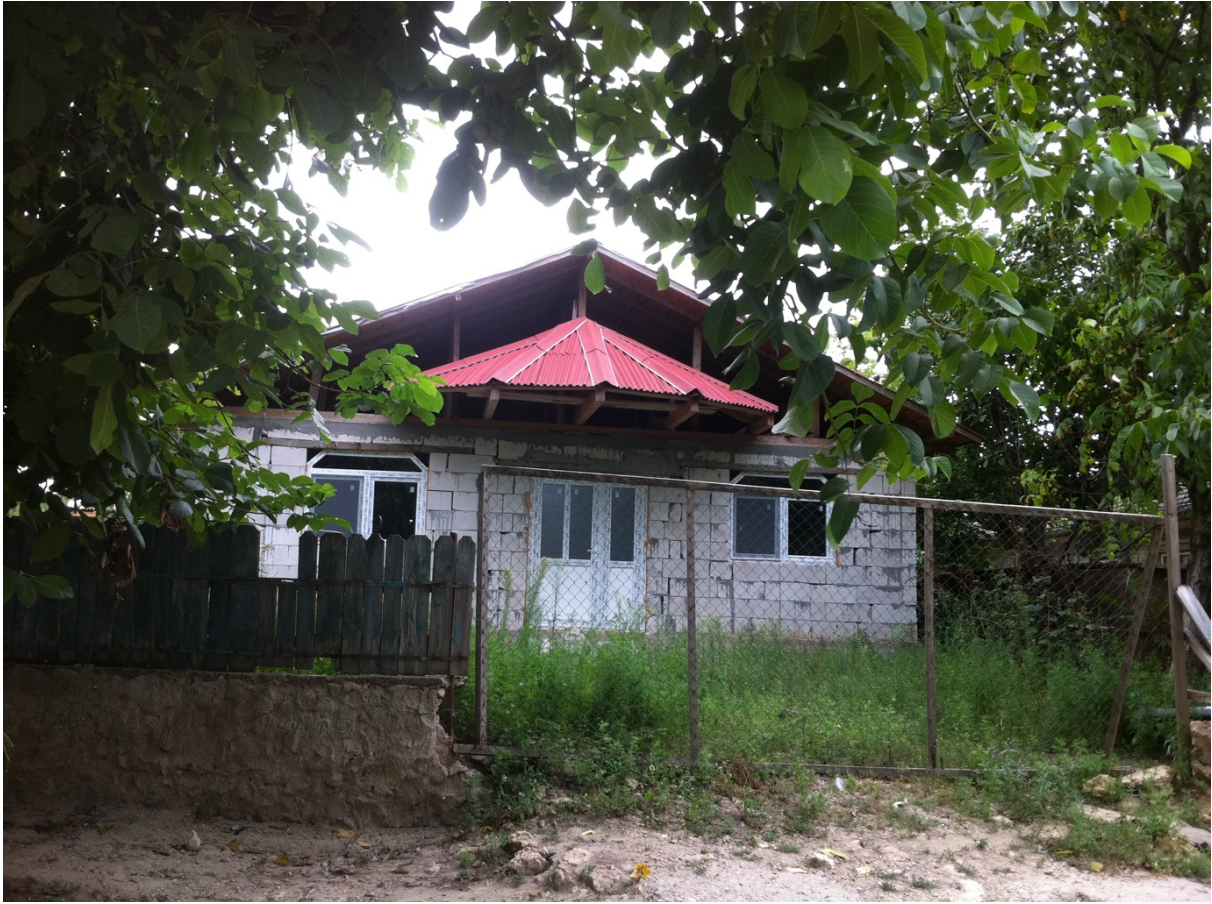
FIGURE 36: House under construction with the first and most important building phase underway
