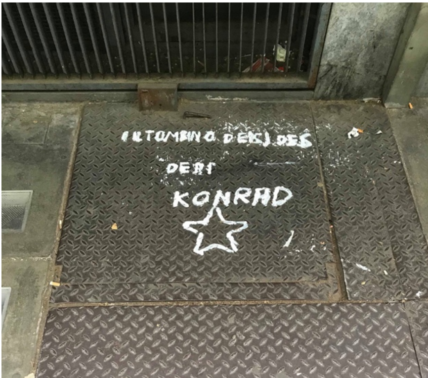
PHOTO 7: The manhole cover where the building's electrical system is found. After that night, it has been 'patrimonialized' by squatters as a place of worship (Photo by Chiara Cacciotti)
